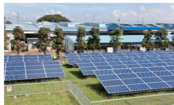
Part of the solar power generation system at the Oyama Factory
